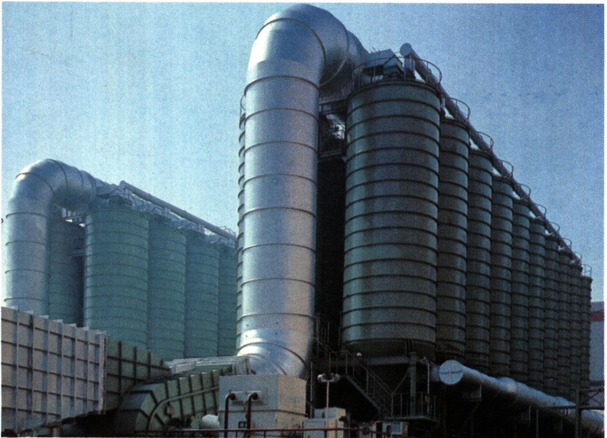
Antipollution equipment at a steel plant. (Courtesy of Nippon Kokan)
